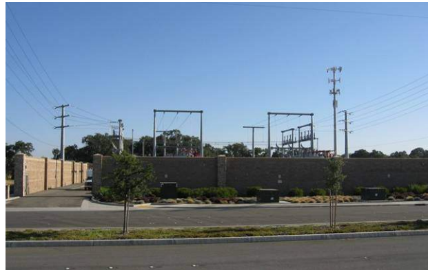
Figure 1 - Roseville Electric's Westplan Substation
