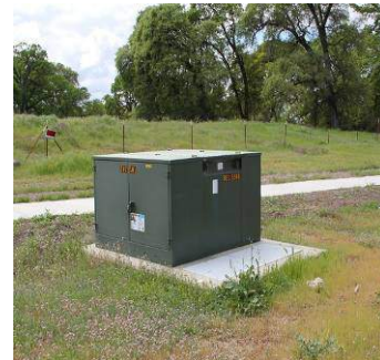
Figure 3 – Main Line Switch
