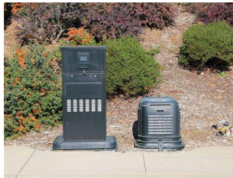
Figure 15 – Comcast Fiber Node and Power Supply
