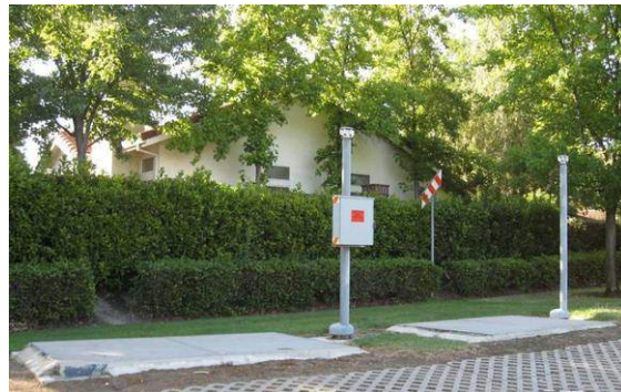
Figure 7 – PG&E Gas Regulator Station, Country Club Drive & Badovinac Drive
