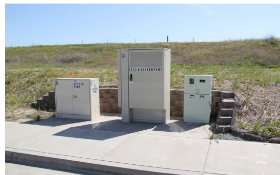
Figure 12 - Electronic Cabinet w-SAI & Pedestal
